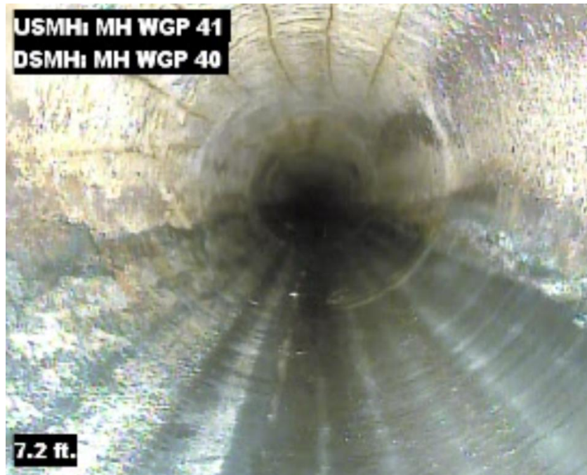
Figure 1 – WGP Interceptor (27-inch diameter reinforced concrete pipe) Pre-rehab video showing severe corrosion and exposed rebar
