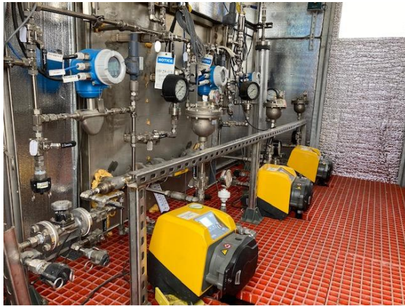
North Dosing System
